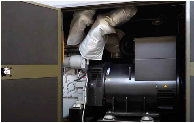
STAMFORD® S6 alternator inside the special canopy
