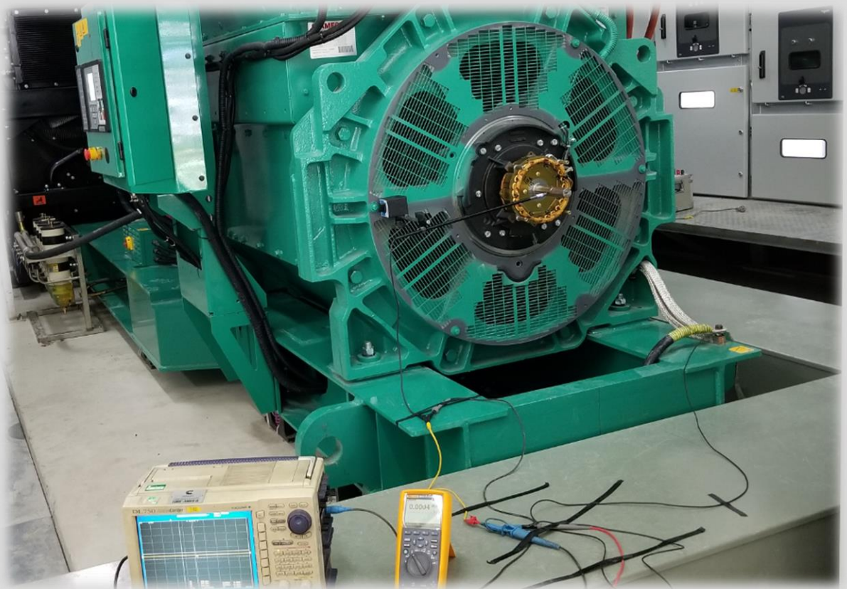
Figure 1: HVSI804S1 Alternator with Shaft Voltage testing apparatus
