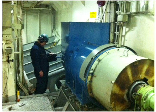
Inside the engine room with a new STAMFORD ® PM7
