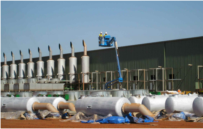
The installation at Christmas Creek followed successful power projects at the Savannah and Cloudbreak mining sites
