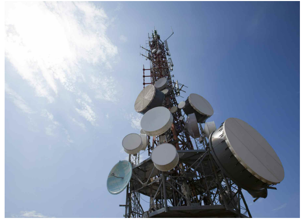
One of the base stations deployed in Saudi Arabia
