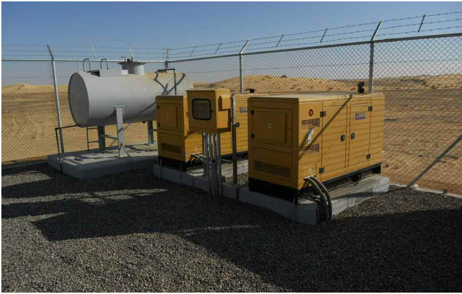
Shanghai Cooltech Power's gensets with STAMFORD® P1 alternators in situ
